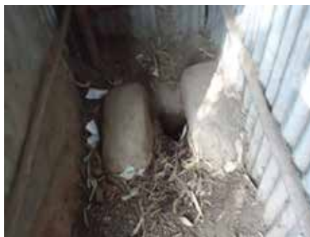
Figure 3 Toilet facilities for girls at Enseno Secondary School, Meskan district, Ethiopia (interior)
