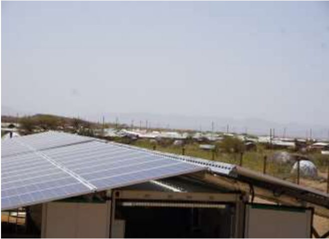
A 44 kW p solar hybrid mini-grid project implemented by NAL Off-grid Limited in Naduat, Turkana County through the RBF support.
