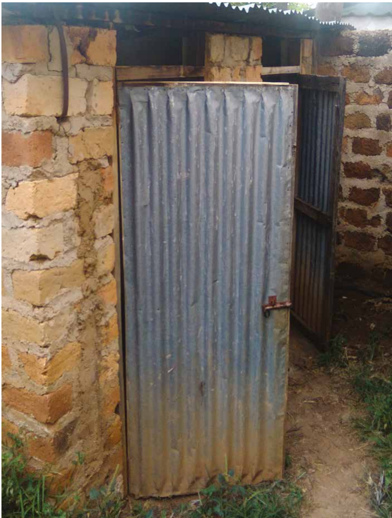
Household toilet facilities
