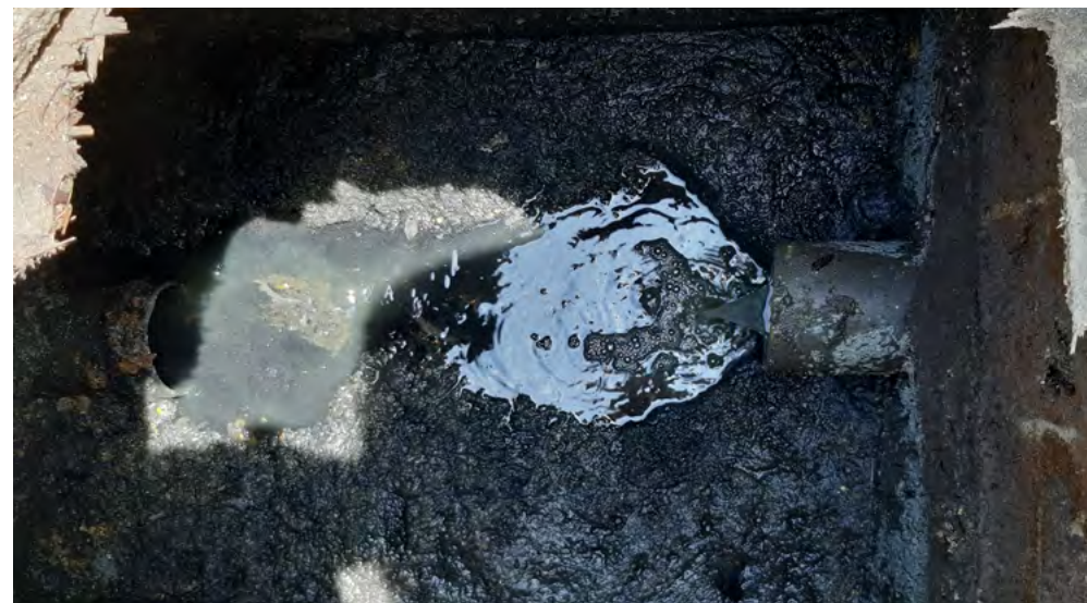
Inlet of the DEWATS
