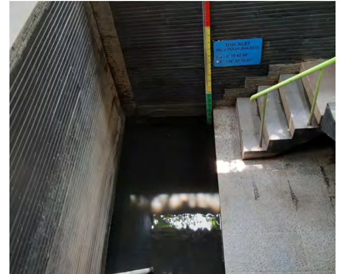
Raw sewage pump station
