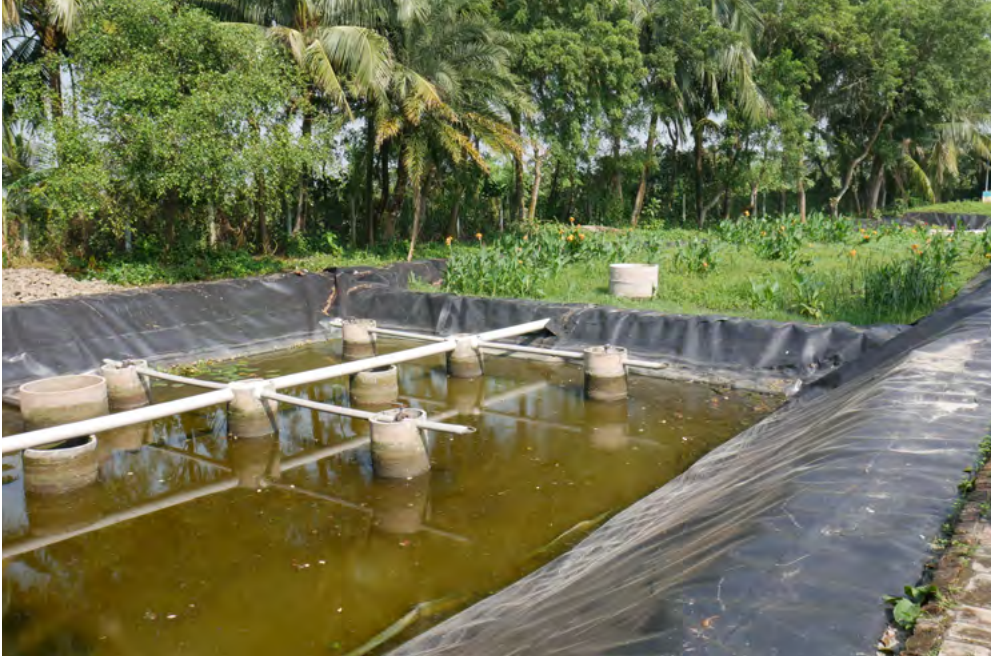
BOD levels of treated water are significantly lower than canal water beside the FSTP
