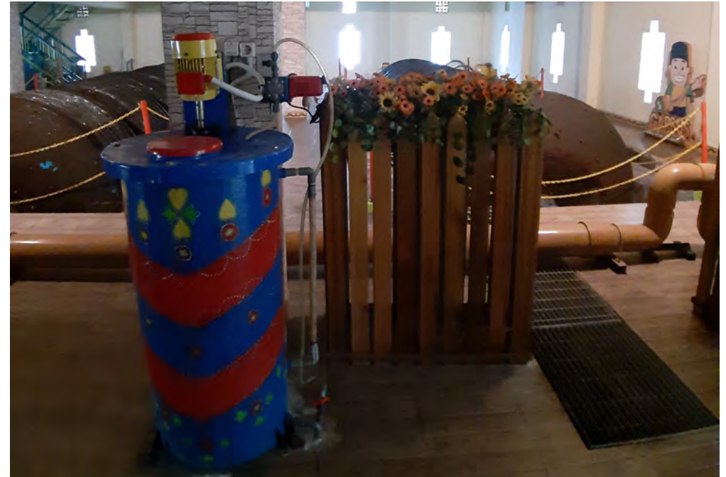
Disinfectant dosing unit, with the final clarifier below the tiles pictured
