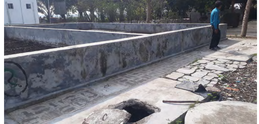
Reserve tanks which drain water from the sludge drying beds
