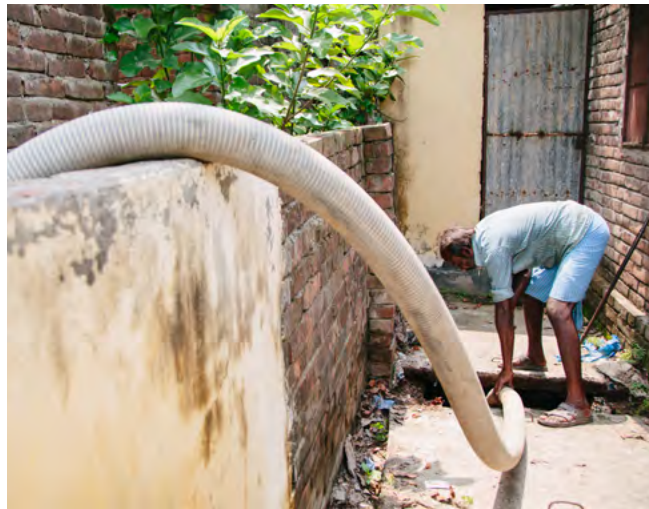
Desludging household containment
