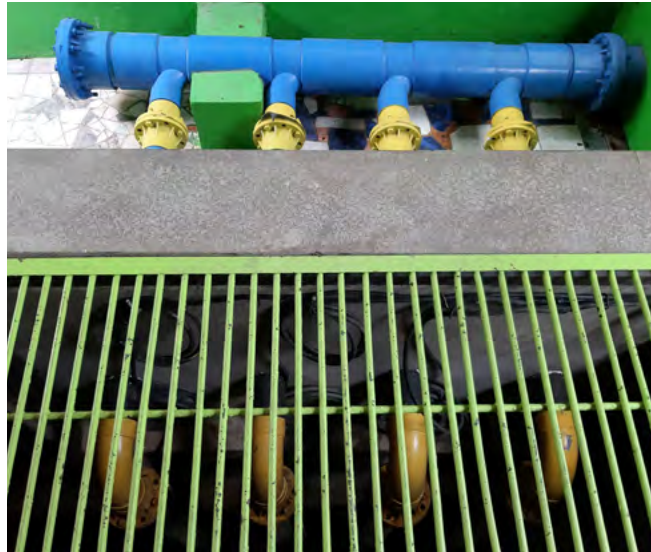
Bar screen with submersible pump
