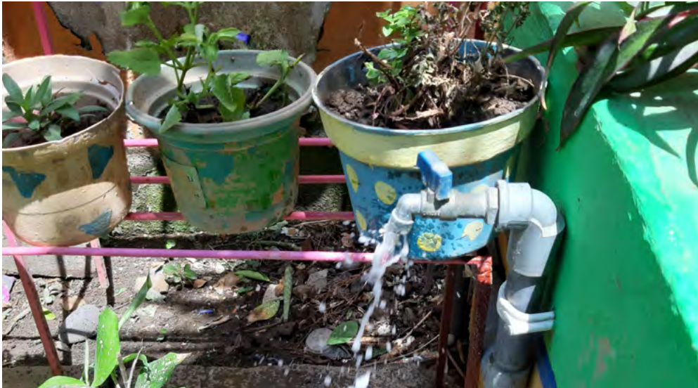
DEWATS tap for reused water in Abbulo Sibatang
