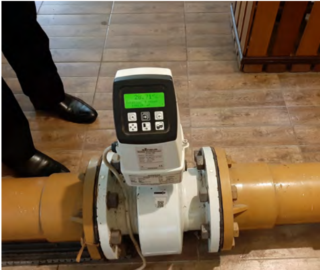
Inlet automatic flowmeter
