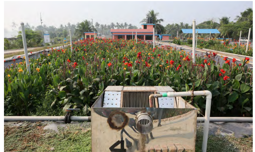
Manual bar screen to remove garbage from sludge discharging into vertical flow constructed wetland
