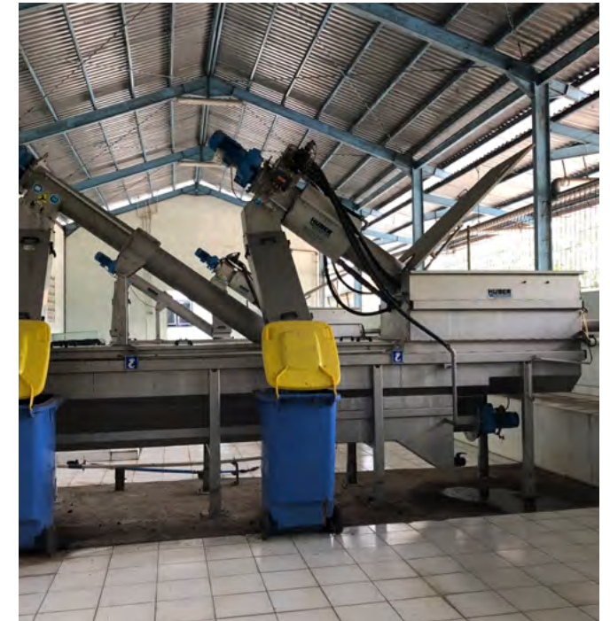
Mechanical sludge screening using Huber acceptance plant
