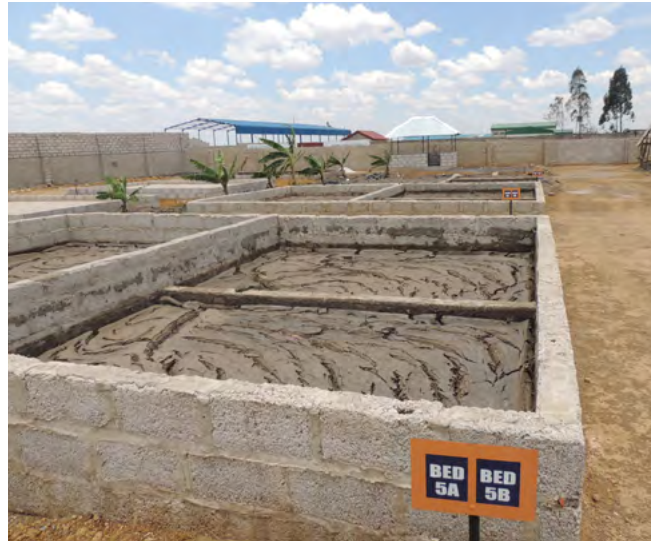
Lined but not roofed drying beds at Kanyama FSTP
