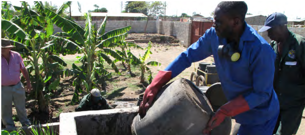
Kanyama FSTP worker emptying sludge
