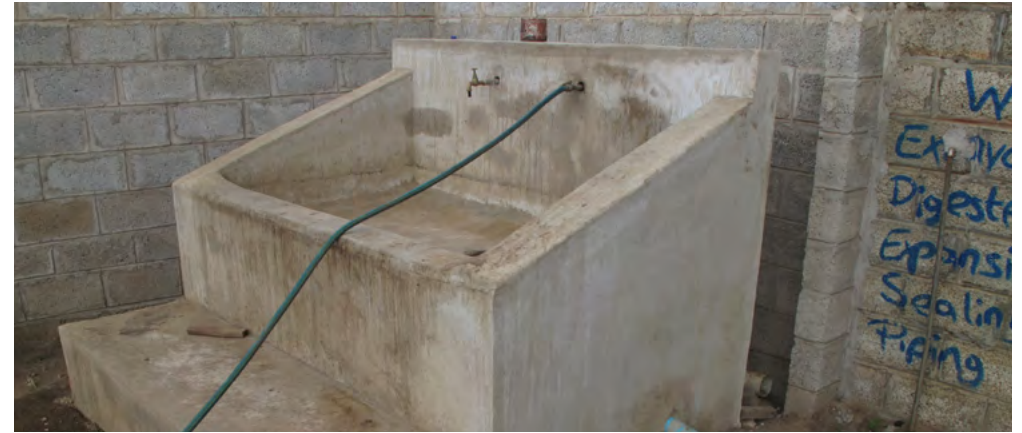
Washing trough for cleaning barrels at the Kanyama FSTP
