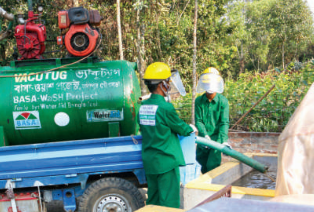
Workers are disposing sludges in the co-compost plant which has collected from different location in the Sakhipur Municipality
