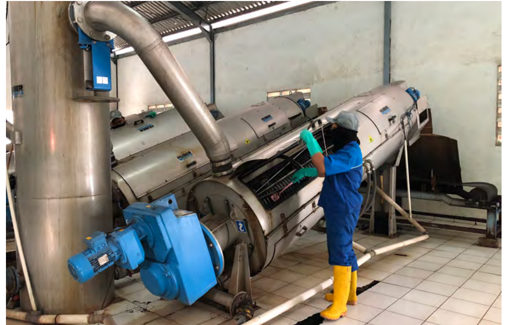
A Huber screw press unit in operation
